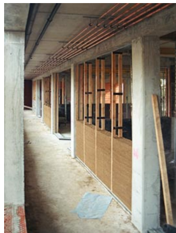
Rammed earth construction of the non-load-bearing walls. Mobile 'slidable' shuttering on timber posts was used and shifted upwards with each new layer of rammed earth.
