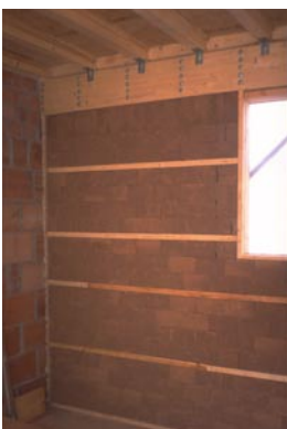
New extension to the Eilberg house with wall construction as stacked wall lining
