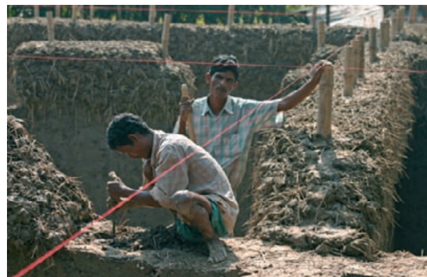
Cob walling built on top of a brick foundation and damp proof course. The wall surfaces are later trimmed flat using sharp flat spades.
